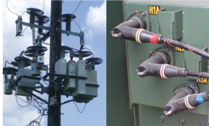
Typical distribution transformers where maintenance and monitoring are critical
